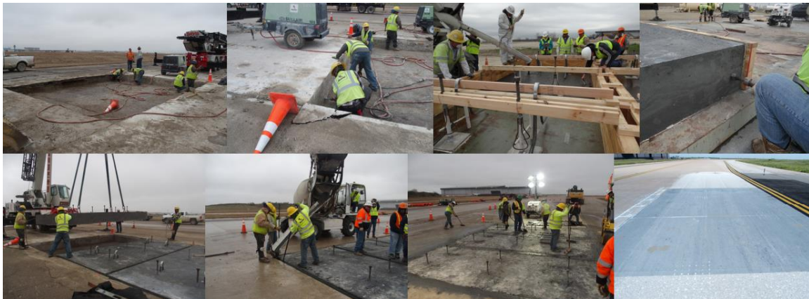
Figure 2-3 Implementing UHPC precast panels, surface roughening, and onsite UHPC joint grouting (Karmacharya et al., 2023)
