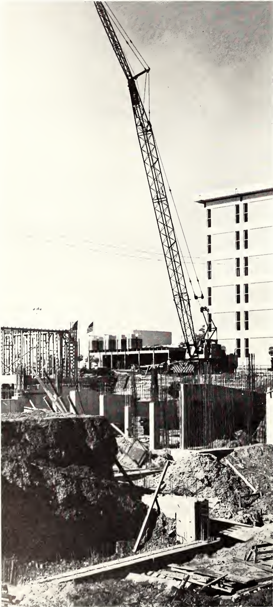
An ice storm in January temporarily stopped construction on Carlisle Hall, a faculty office building going up between Ransom Hall and Preston Hall. A walkway beneath will make the six-floor building eight stories high and the tallest structure on campus.
