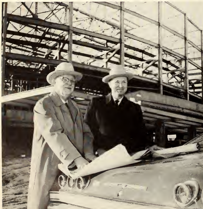
Barnes and then-president Dr. Jack Woolf inspect construction of Texas Hall in 1965.
