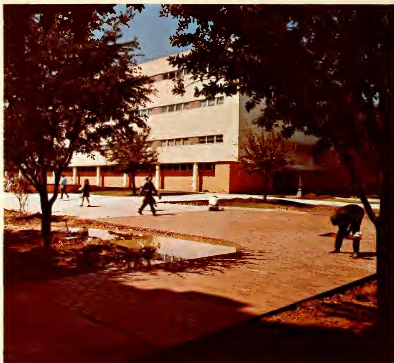
Workmen add finishing touches to brick sidewalk replacing the old intersection of College St. and Second in front of Engineering Building.
