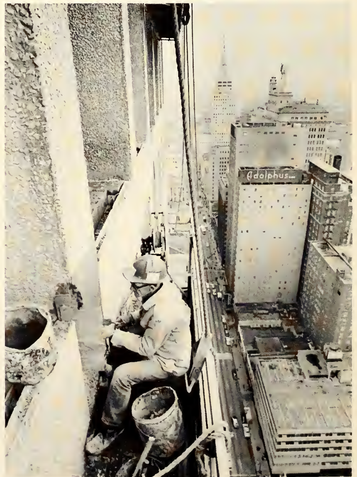
A workman, putting the finishing touches on the exterior of One Main Place, rides high over the Dallas skyline.
