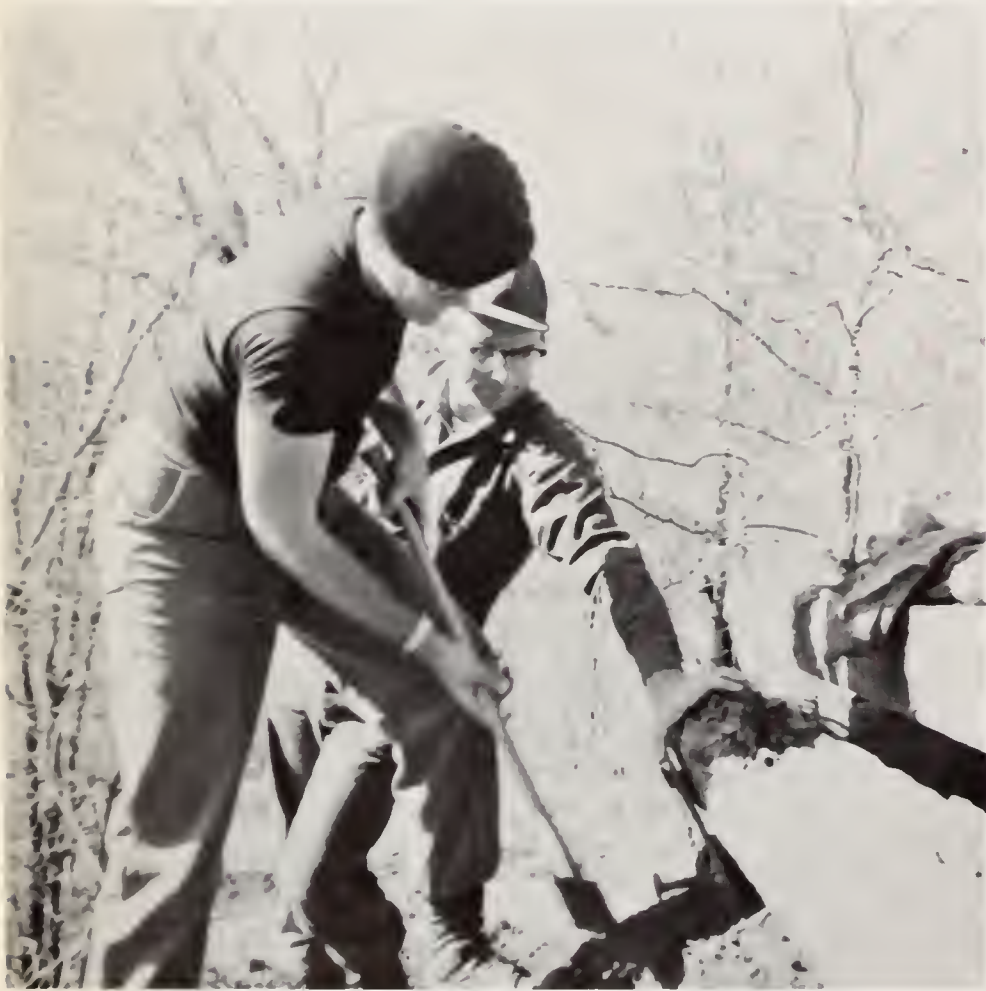
Digging trenches and repairing bunkers hit by enemy shells are jobs an insurgent Cadet learns, as two team members show.
