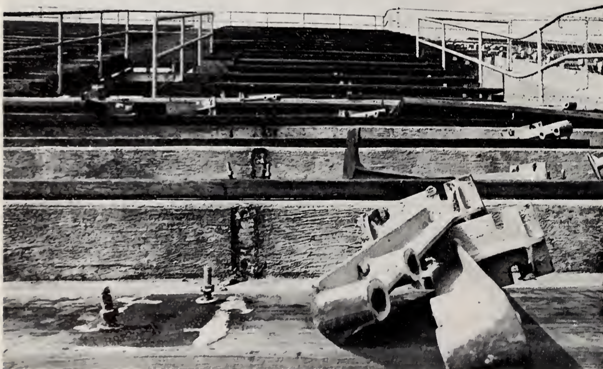
RIGHT, ABOVE: Memorial Stadium comes down to make room for the new student activities building. TOP: Bud Elliott.
