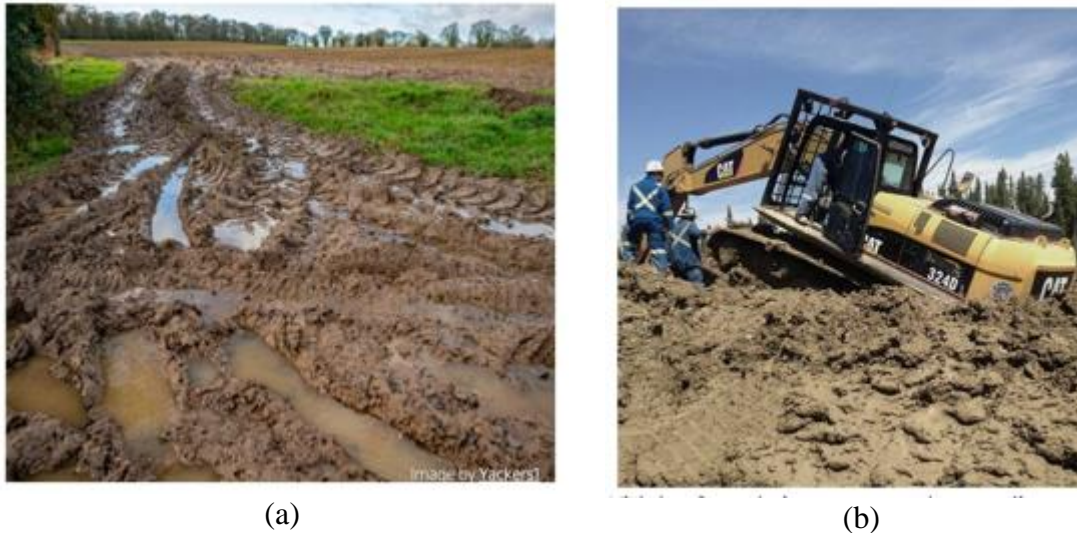
Figure 2-4 (a) Weather variation consequence of weak soil; (b) Construction equipment sinking in weak soil
