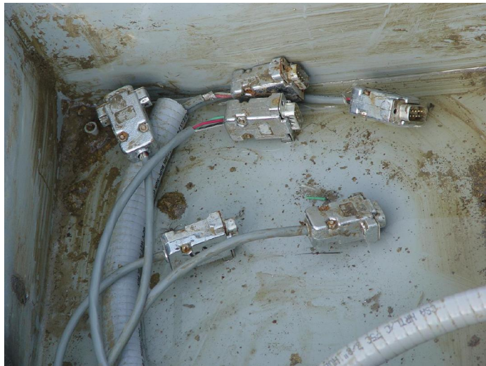
Figure 4.10 DB9 Pins Rusted
