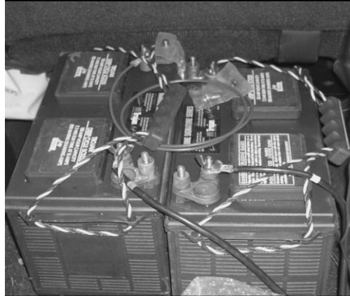
Figure 3.3 Two 12 V each deep cycle batteries
