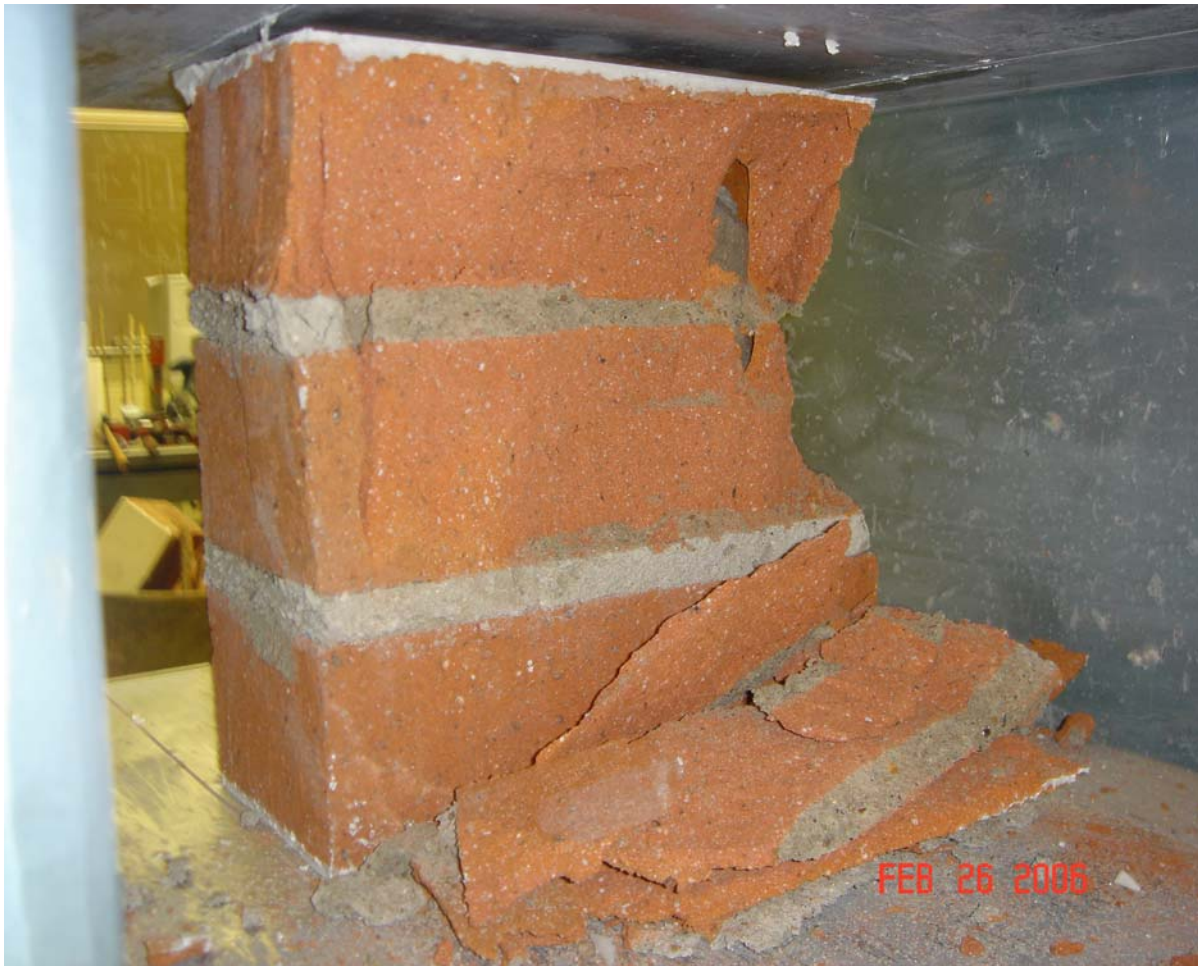
Figure 3.37: Prism with Approximate h/t Ratio of Two Built with Brick “C” and Type N Mortar Exhibiting Signs of Conical Mode of Failure.
