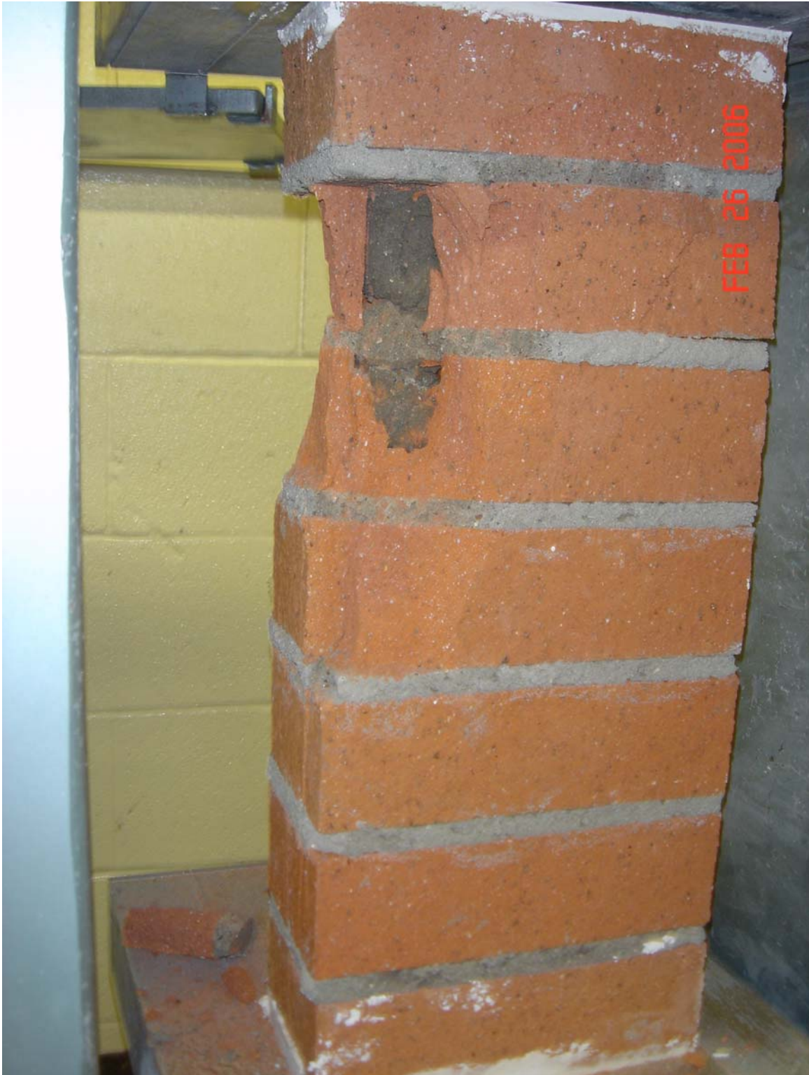
Figure 3.40: Prism with Approximate h/t Ratio of Five Built with Brick “C” and Type S Mortar Exhibiting Signs of Vertical Splitting and Face-Shell Separation Modes of Failure.
