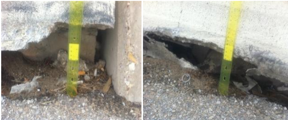
Figure 5.11 Close view of vertical displacement at SH 360 - Control Section
