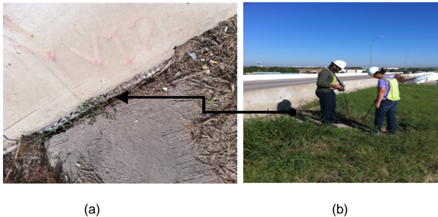
Figure 5.3 (a) Horizontal movement seen near V2 location (b) Testing at V2 location
