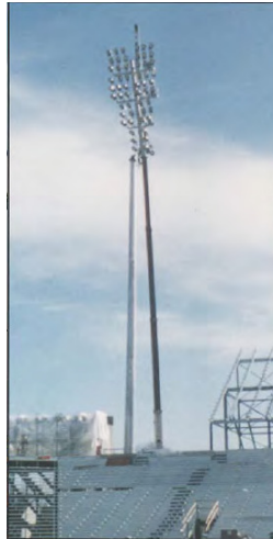
Figure 1.6 A Sports Lighting Tower[11]
