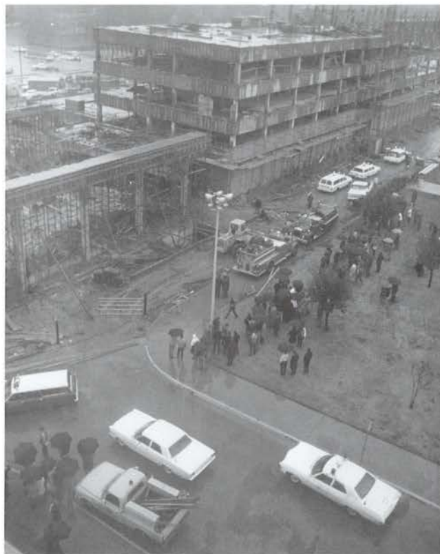
7.11 One of the few construction accidents at UTA occurred in 1970 when, during the construction of University Hall, the freshly-laid concrete roof of the theater collapsed. While the incident attracted much attention, there were no serious injuries.
