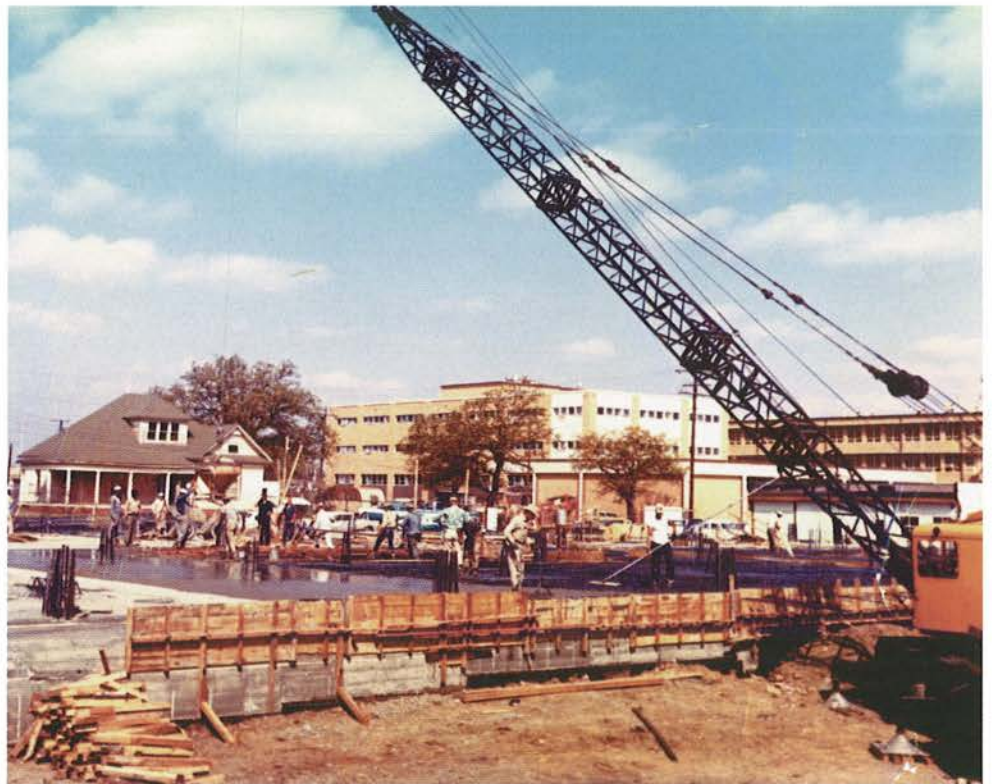
6.6 As the ASC campus expanded south and west along Cooper Street, some Arlington residents found themselves in the way of the school's progress. When the library's foundation was poured in 1962, a wood-framed house stood directly in front of the construction and beside the Science Building.
