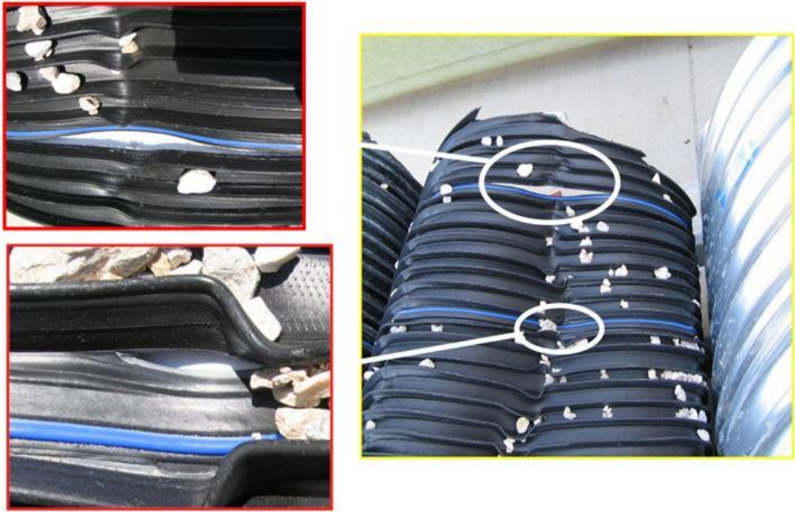
Figure 3.39 Tearing of HDPE Part at Joints
