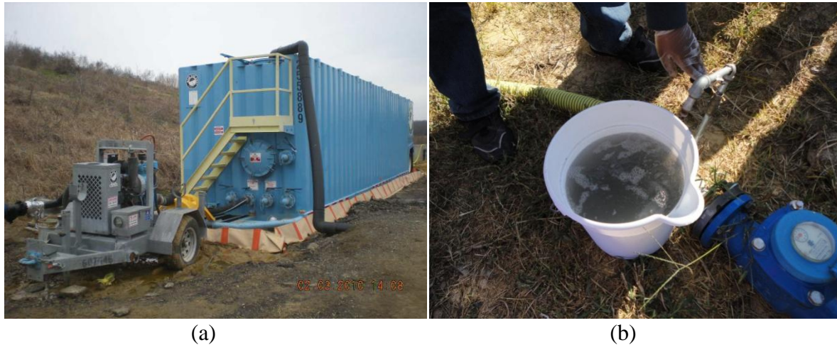
Figure 3.18 (a) Leachate Storage Tank and (b) Leachate Collection
