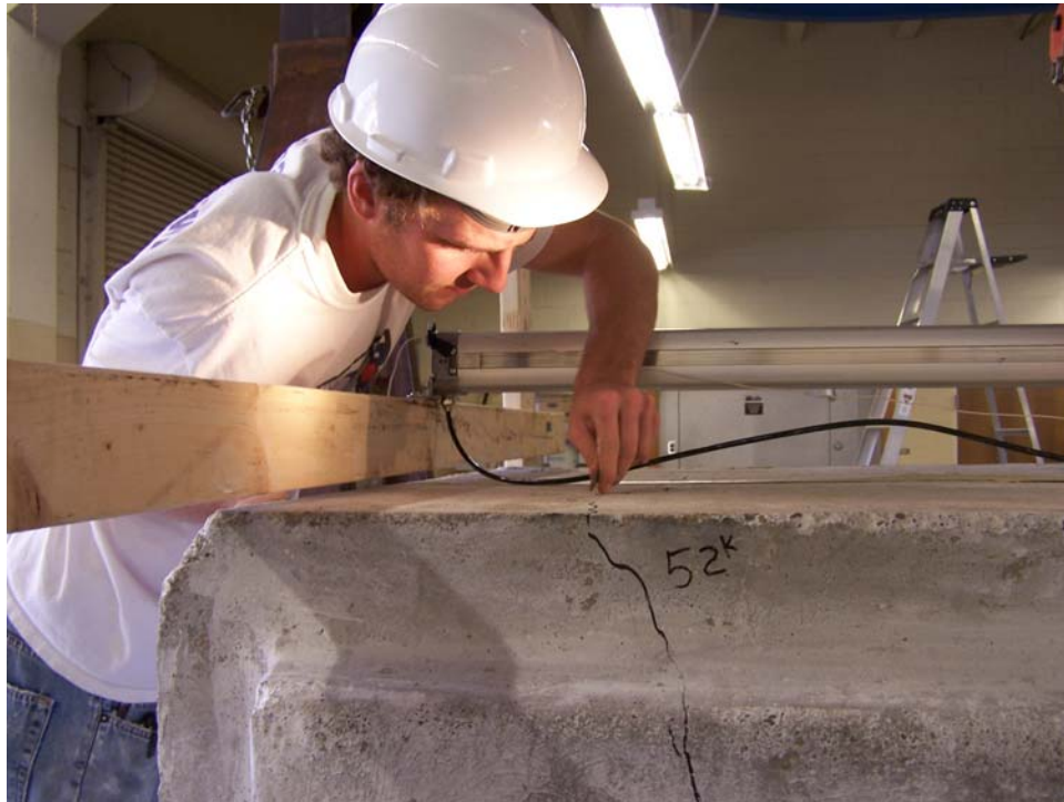
Figure 2.19 Crack Monitoring Process
