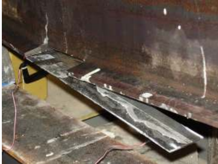
Figure 3.19: Failures with de-lamination and tearing of beam
