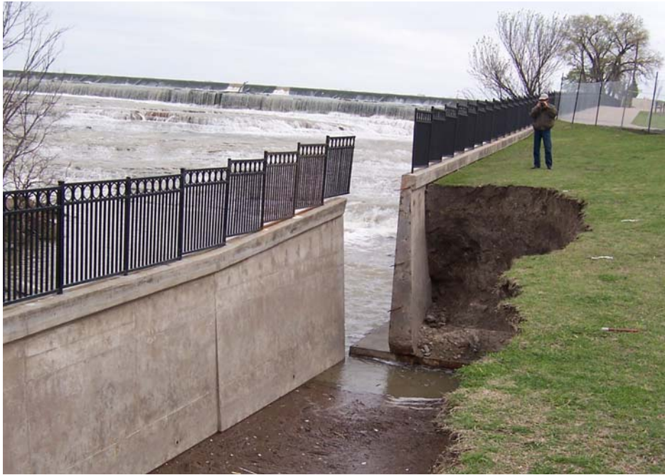
Figure 1.1 – Wall Failure Along Dam Spillway
