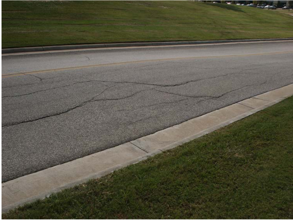
Figure 2.3 – Pavement Heave and Cracking
