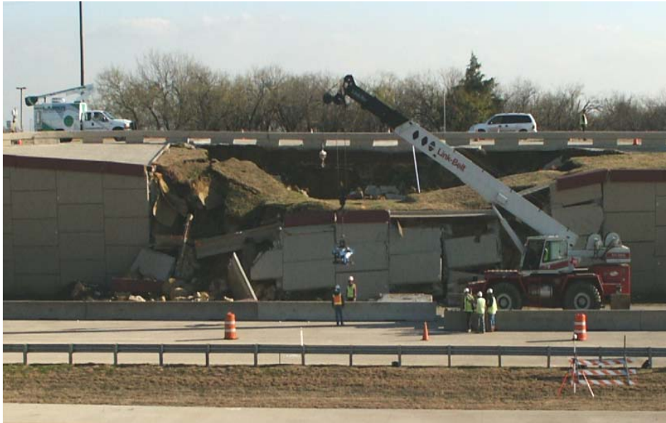
Figure 1.2 – MSE Wall Failure Along Highway
