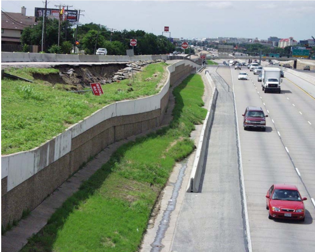
Figure 5.6 – Local MSE Wall Failure Due to Sliding (photograph courtesy of Paul Spraggins, PE, TxDOT Central)
