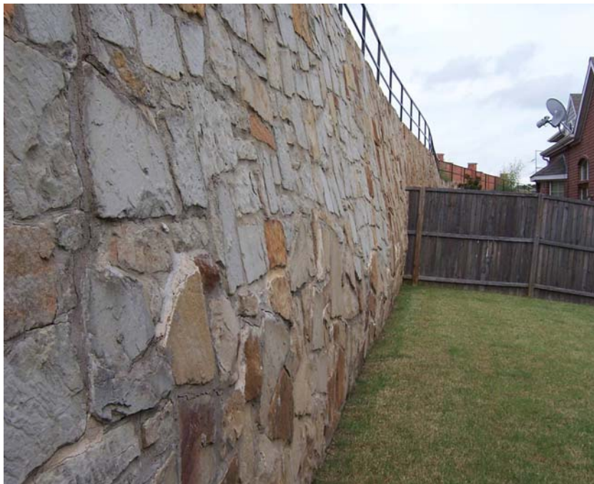
Figure 1.4 – Severe Wall Distress. Note bulge at bottom.
