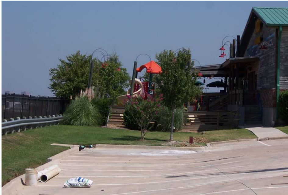
Figure 1.3 – Severe Wall Distress (wall at left). Note rotated light standards, deformed guardrail, sunken pavement and curb separation.
