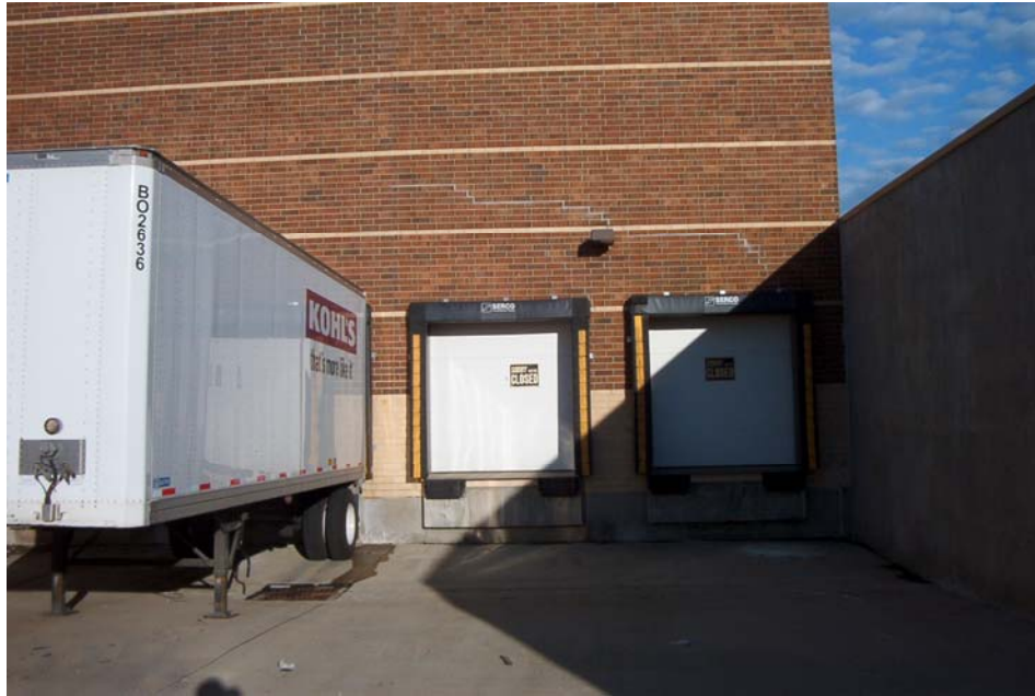
Figure 2.5 – Brick Facia Cracking
