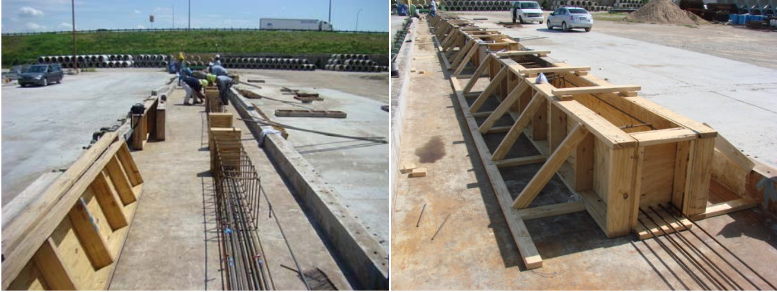
Figure 3.28 Typical photos of reinforcement caging and formworks in the third phase study
