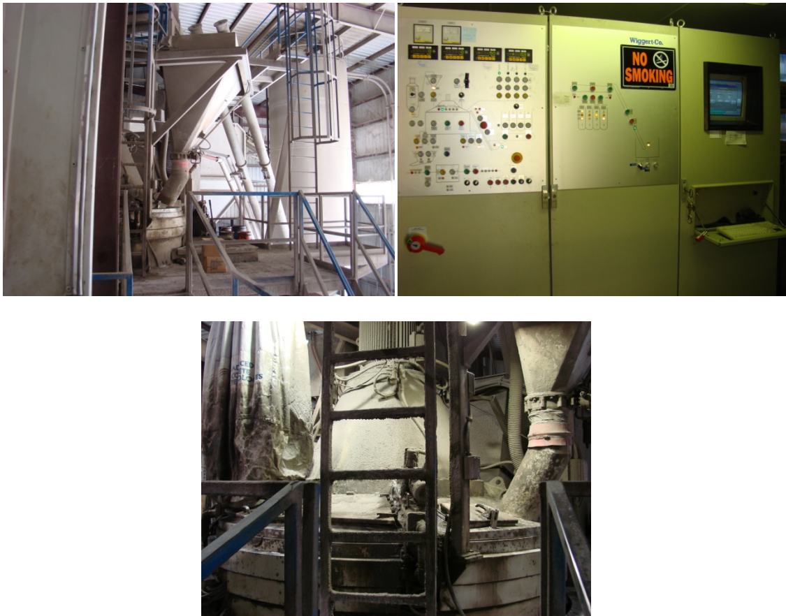
Figure 3.4 Concrete mixing facilities in Hanson Pipe & Precast
