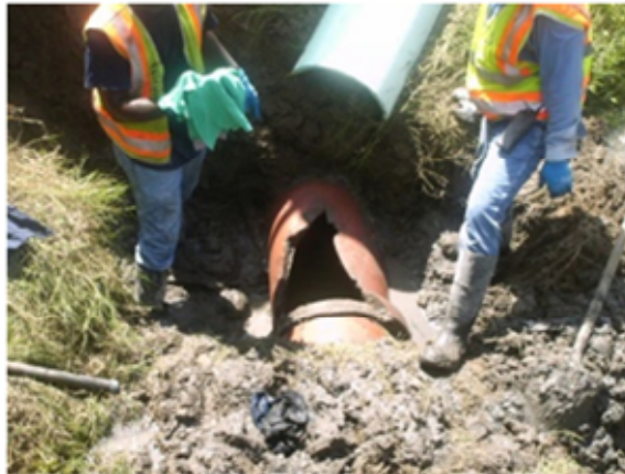
Figure 7.4 Instantaneous Failure (Backhoe Damage) Source: City of Rowlett
