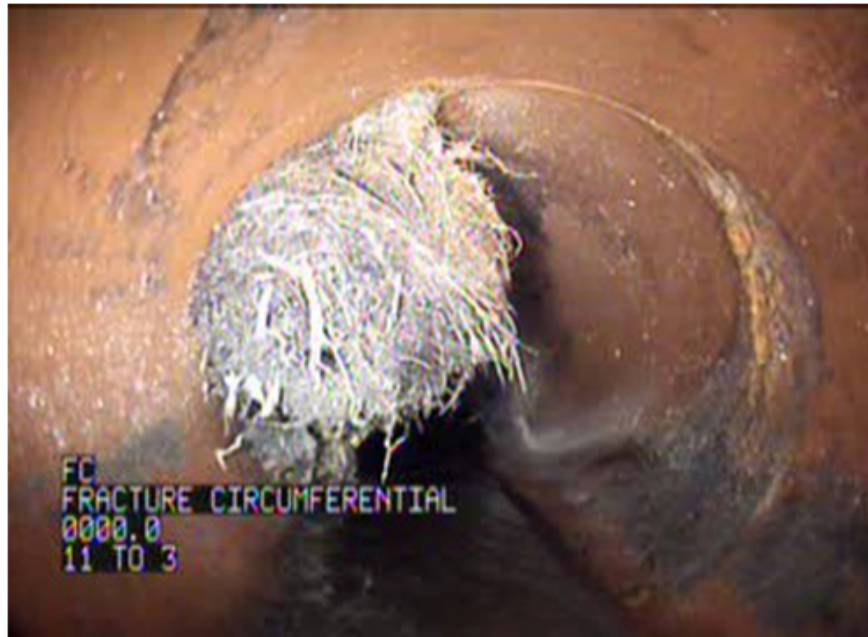
Figure 7.2 Static Failure (Root Intrusion) Source: Forbes, 2010
